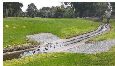
Many a ball was lost in this fast-flowing drain. It didn't deter the ducks though!
